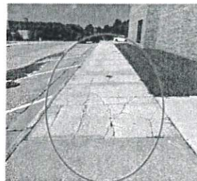
High School west sidewalk. Recommend considering replacement of damaged concrete to prevent possible tripping falls.
